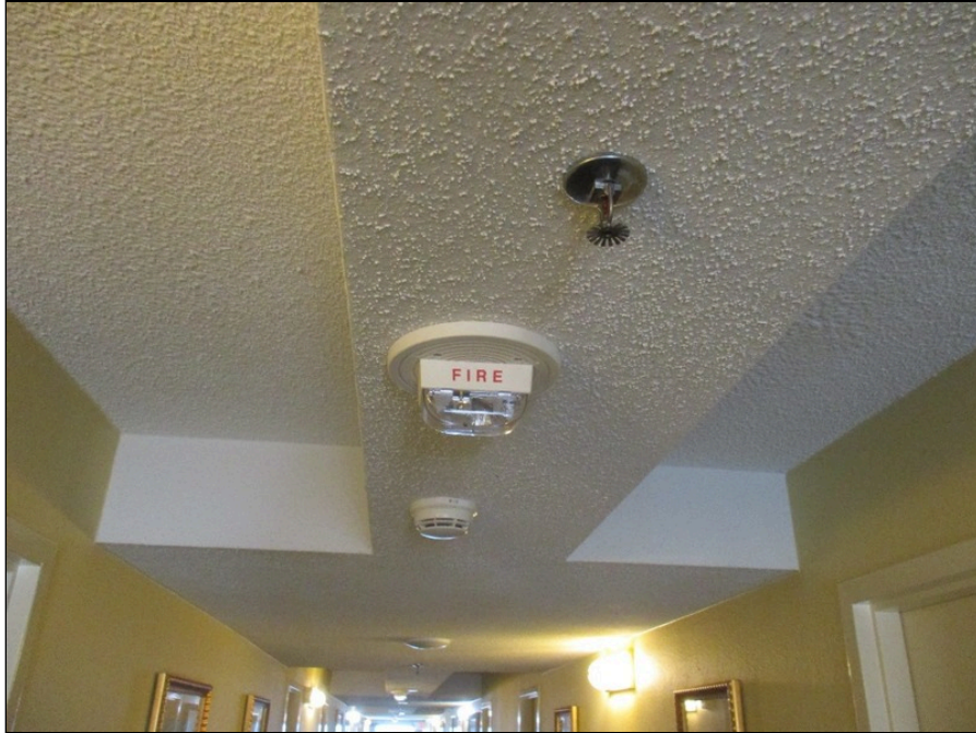
27 - Typical fire alarm and sprinkler head
