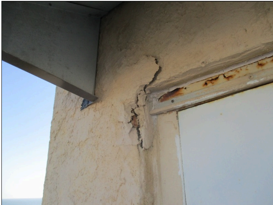
8 - Cracking distress at doorway
