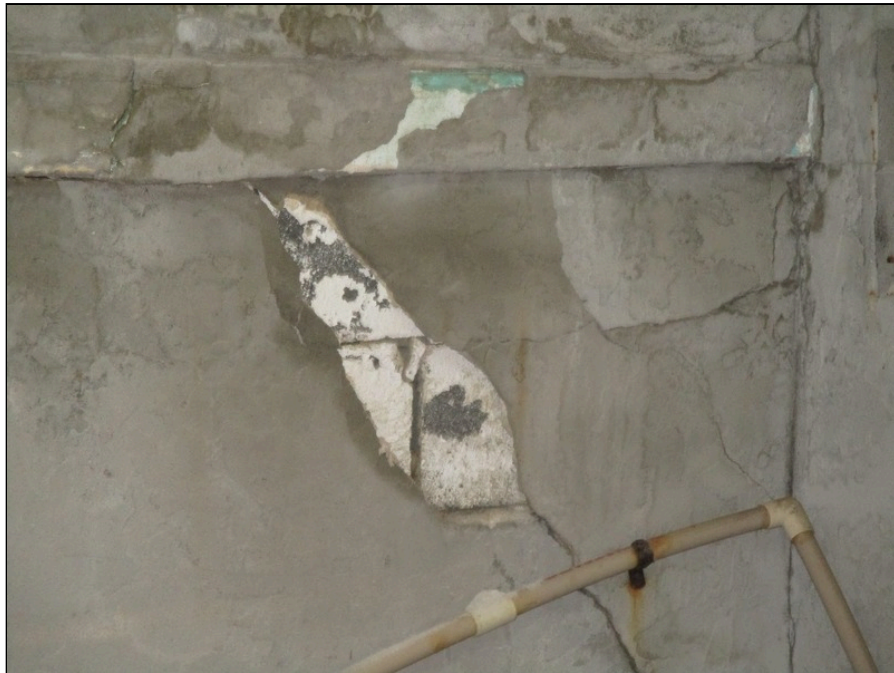
10 - Cracking in pool room exterior wall
