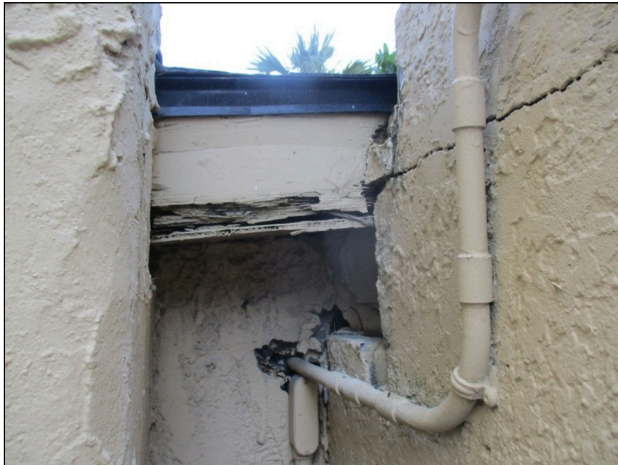
18 - Pool equipment building exterior deterioration
