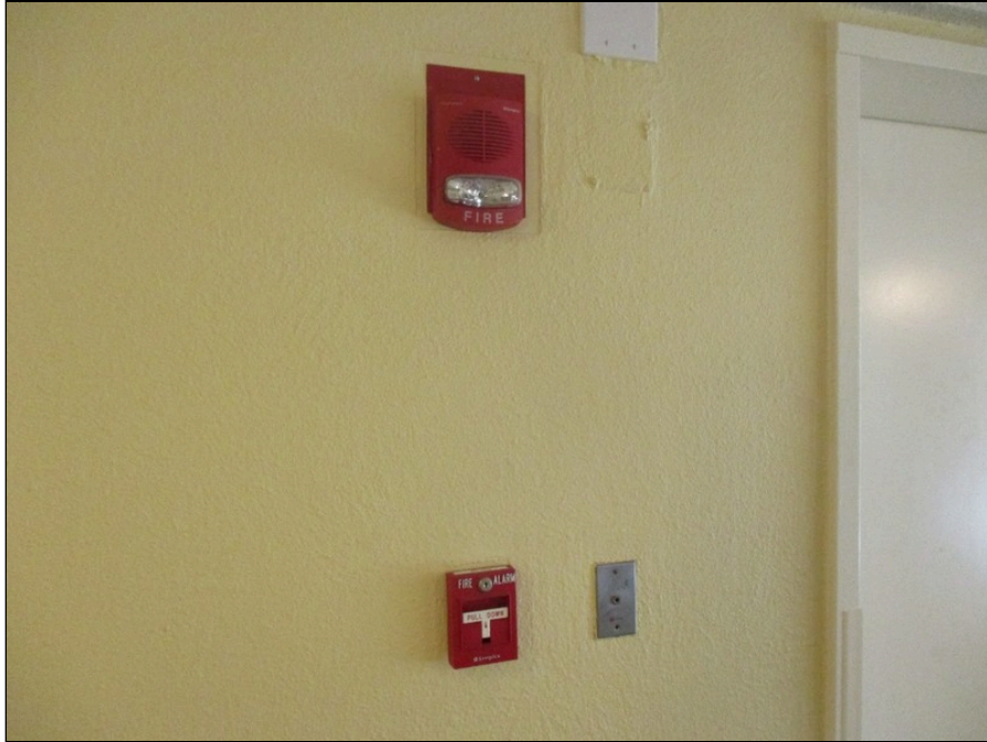
19 - Typical fire alarm and pull station
