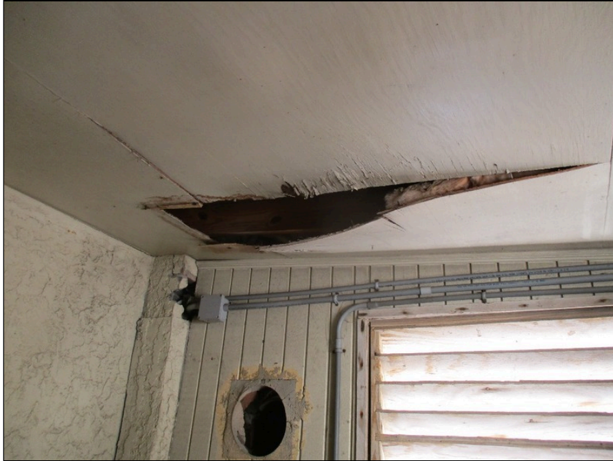
11 - Pool room ceiling deterioration
