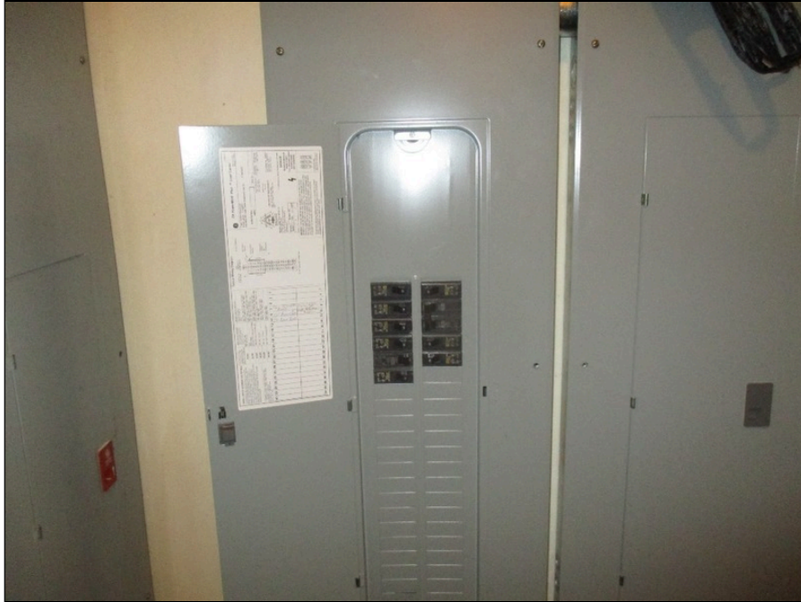
31 - Typical electrical panel
