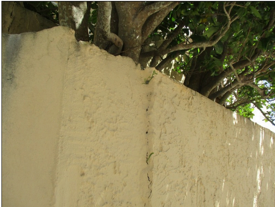
14 - Cracked retaining wall south of Tides
