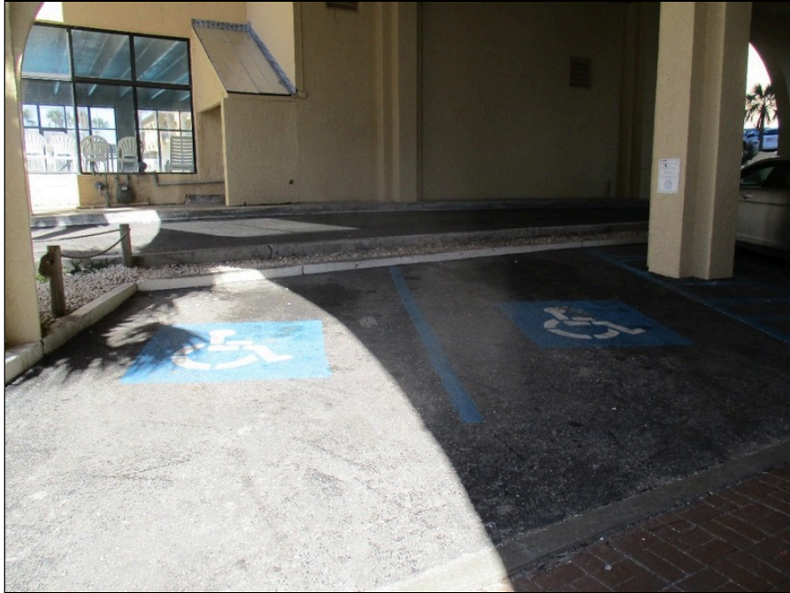
55 - Accessible parking in main service drive - no signage
