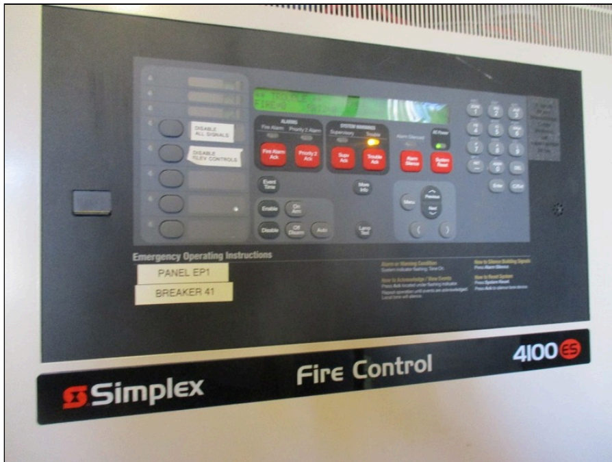
44 - Fire control panel
