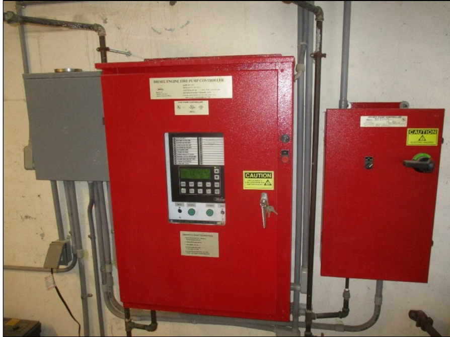
43 - Fire pump controller
