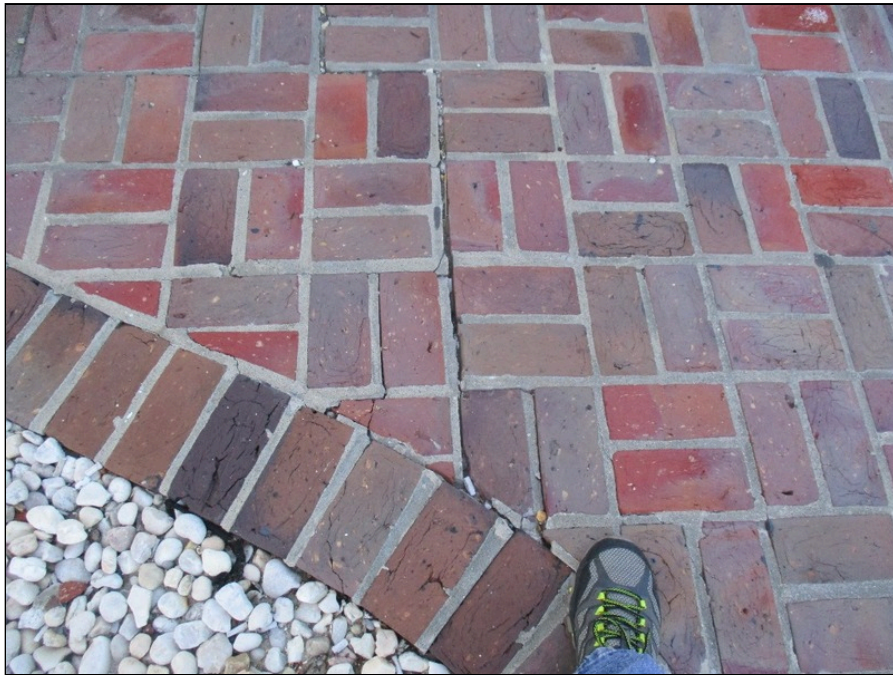
52 - Pool deck brick cracking
