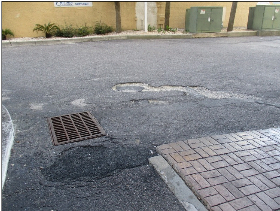
16 - isolated pavement distress, drop inlet
