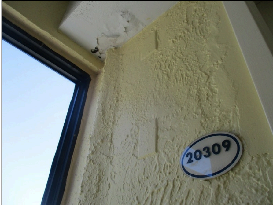
13 - Isolated moisture infiltration at hallway exterior window
