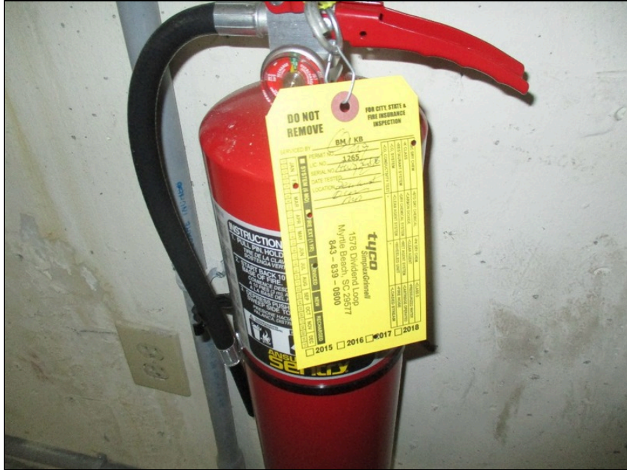
41 - Typical fire extinguisher
