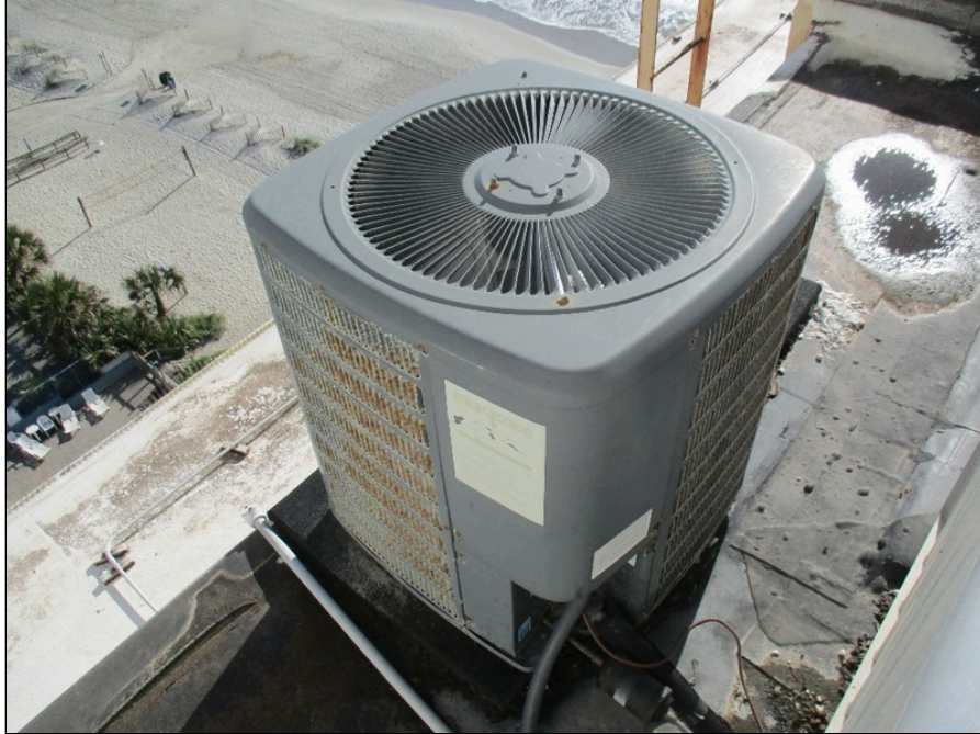
35 - HVAC mounted at Tides lower roof edge
