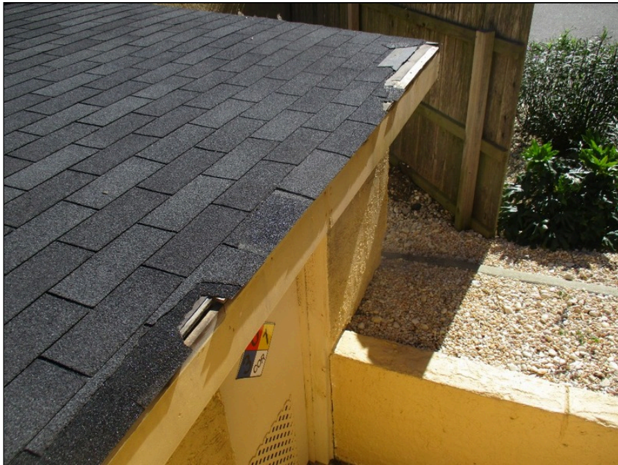
24 - Pool equipment room roof deterioration
