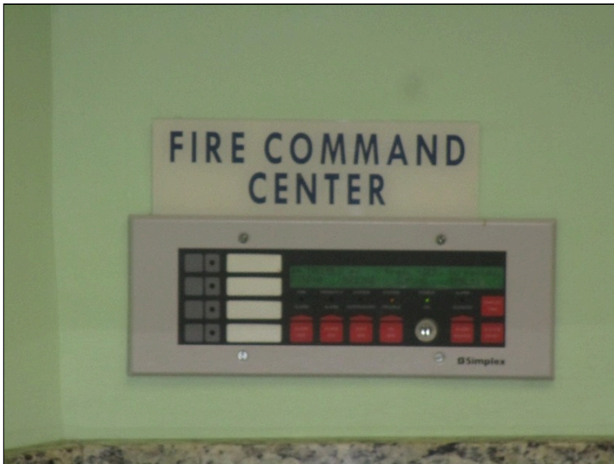
46 - Fire annunciator in lobby area
